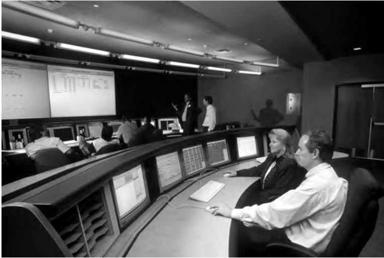
FIGURE 20.1 Manitoba Hydro Control Center in Winnipeg, Manitoba, Canada. (Photo used with permission of ALSTOM ESCA Corporation, Bellevue, WA.)
